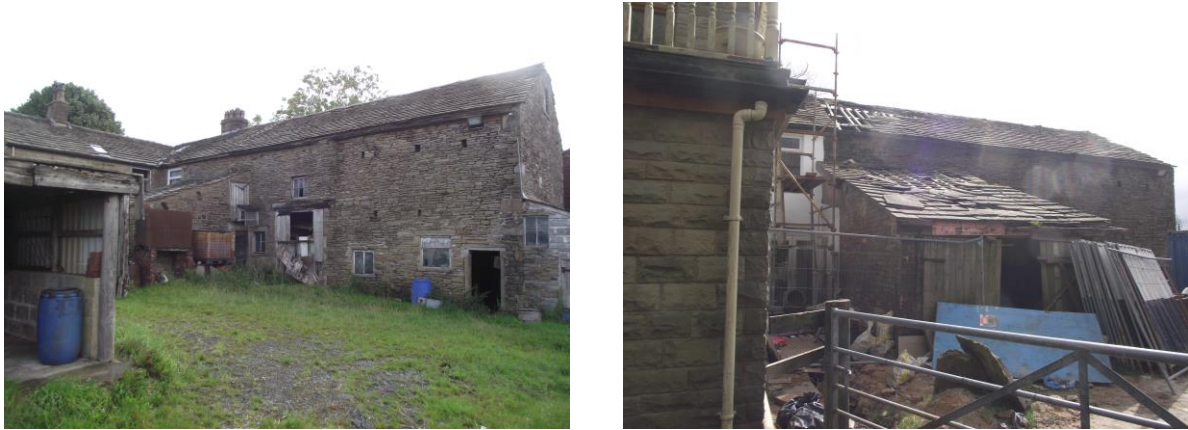
North elevation, above. The windows to the left of the lean-to belong to 475 Blackburn Road. Proposed alterations, over.
